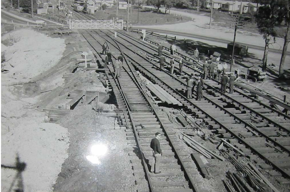
Fig 5. Showing the level crossing and works commenced for the road underpass in 1961.
