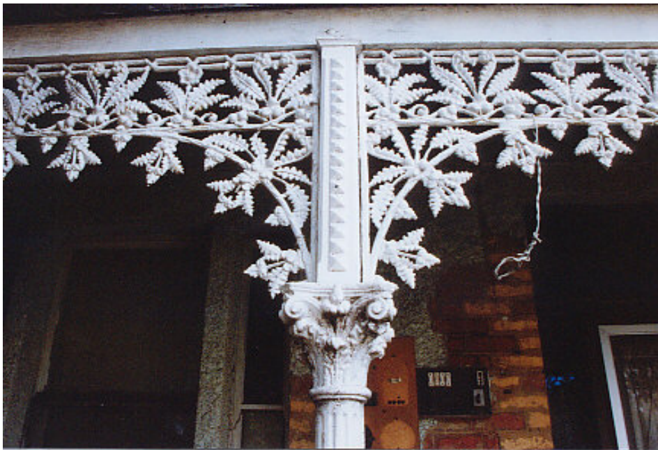
Fig 32 Architectural detail: cast iron valance and brackets in fern design with Corinthian columns. 20 Butler Street. Source: Lorraine Huddle 2000.
