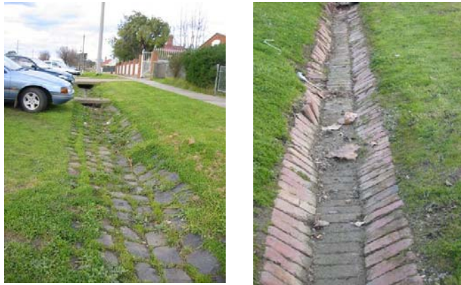
Fig 21. High Street bluestone spoon drain on the left and brick spoon drain on the right. Source: Lorraine Huddle 2003.
