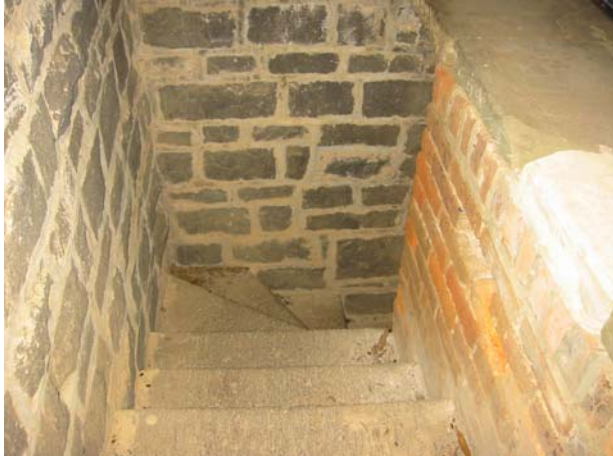
FIG. 24. View of staircase showing bluestone and brick walls, and winding bluestone steps. Source: Lorraine Huddle 2003.
