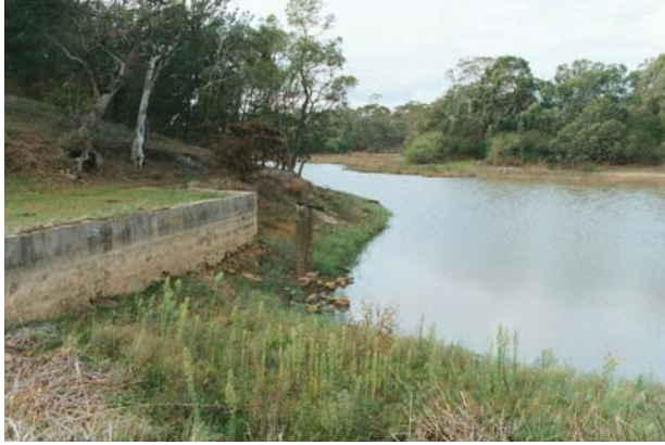
FIG. 17. 1950s concrete wall at the diving end, clearly visible in the drought conditions. Source: Susie Zada 2003.
