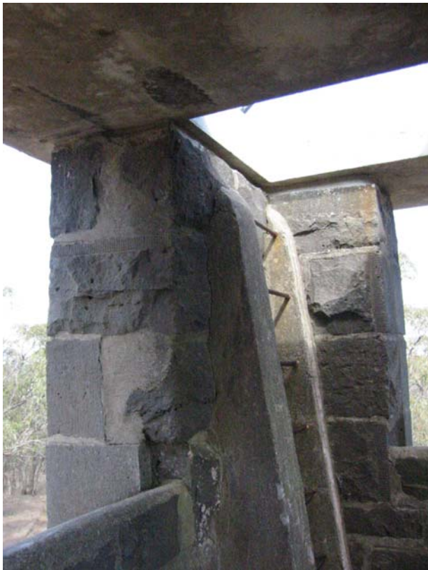
FIG. 25. View of concrete and metal ladder to roof of tower. Source: Lorraine Huddle 2003.
