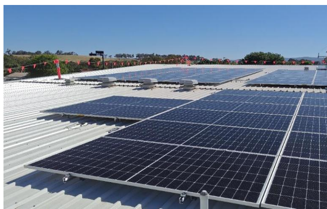
Solar panels on pavilion at Harley Hammond Reserve, Broadford
