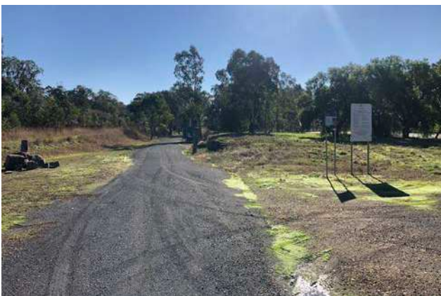
Figure 14: Trail surface was in good to excellent condition for the majority of the trail.
